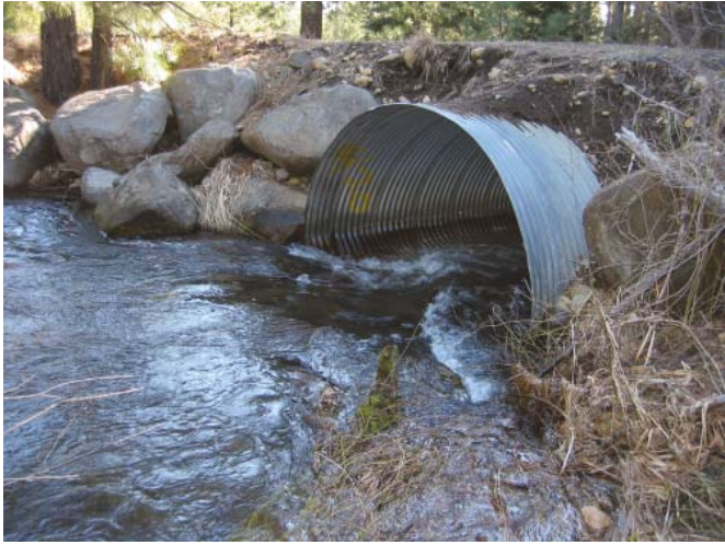
THIS SUMMER, WE WILL REPLACE THIS CULVERT AT THE METOLIUS PRESERVE TO IMPROVE FISH HABITAT. PHOTO: STAFF.
