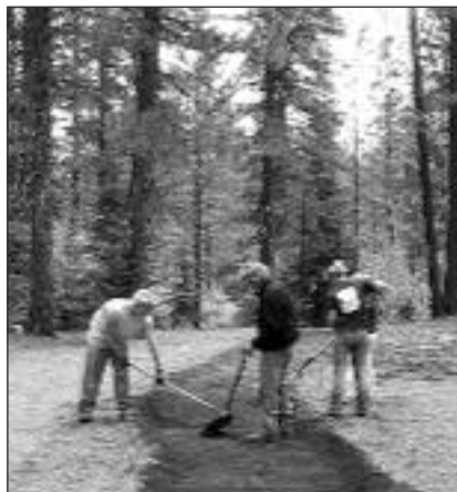
Central Oregon Intergovernmental Council crew members work on the new interpretive trail.
