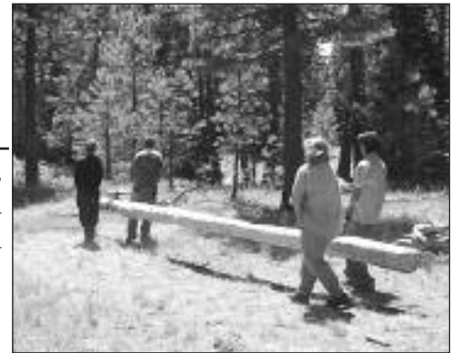
Heart of Oregon Corps crew members constructing boardwalks and bridges at the Metolius Preserve.
